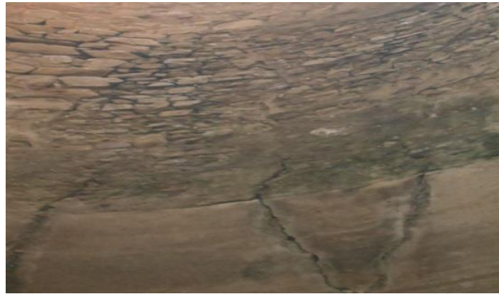
c. The Destroyed wall of well at Agrasen ki Baoli
