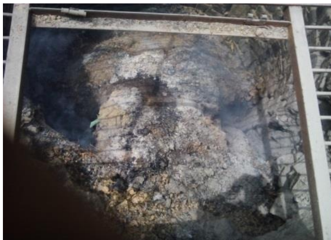
Figure 9 – Dried and extinct well of Kutub ki Baoli Source: Primary survey.
