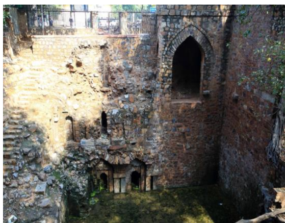
Figure 10 – a. ruined stairs of Hindu Rao ki Baoli Source: Primary survey
